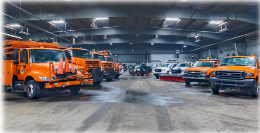
Skylights in the DPW garage help to conserve energy on sunny days
