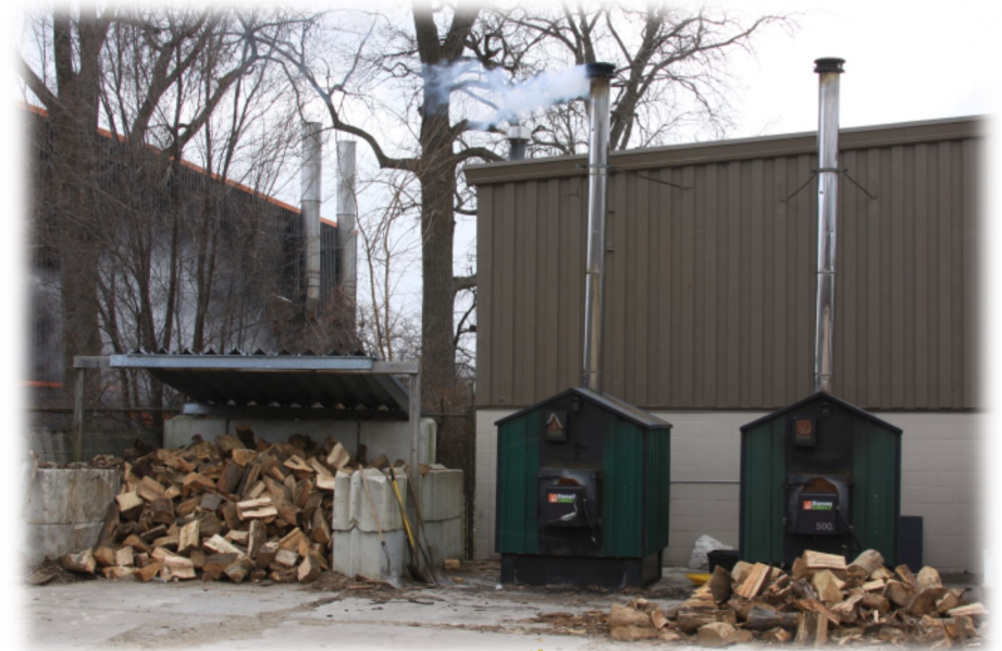
Wood burner located at Oak Park Department of Public Works
